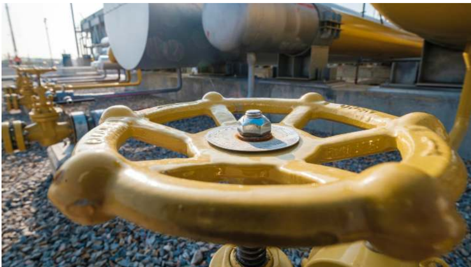
>> A compressor station on the Southern Gas Corridor
